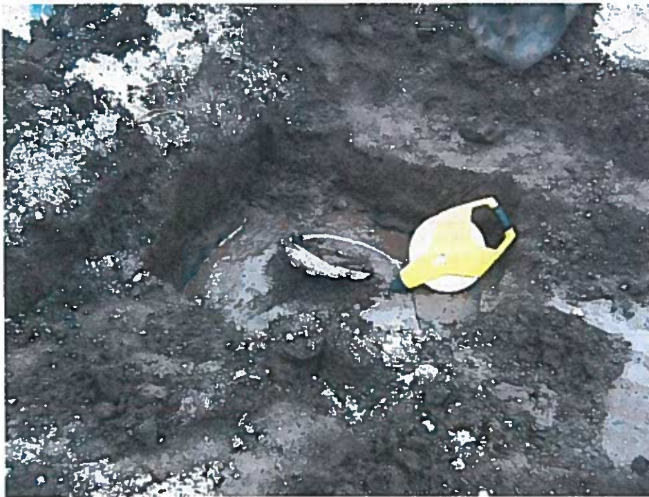
View of the uncovered leak in the bypass basin from the detection survey.
