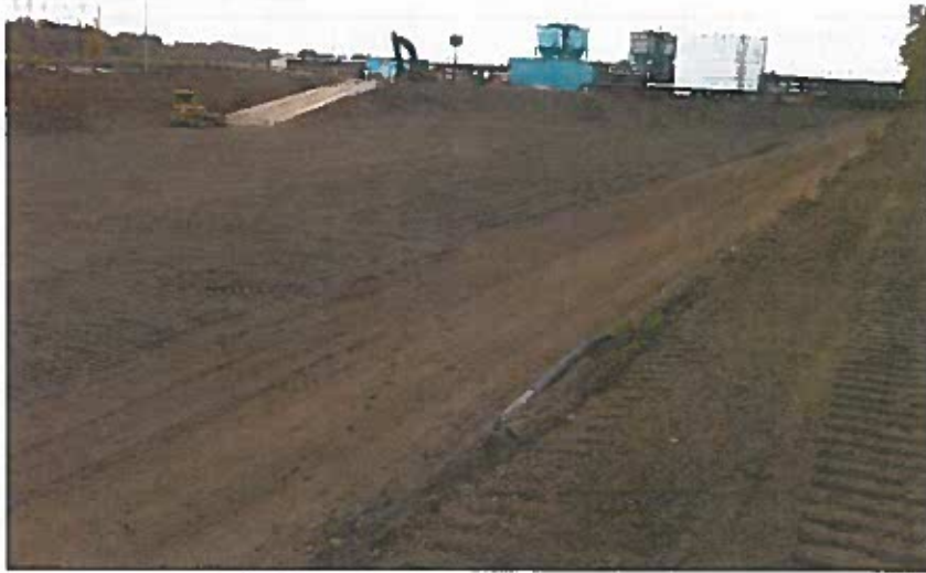
View of basin subgrade from the northwest corner of the basin facing southeast. Note concrete aprons and hypalon removed.
