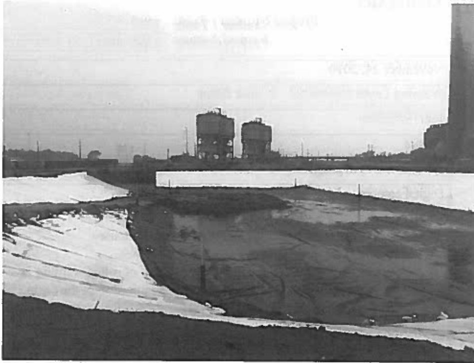
View of partially placed cushion layer in southern portion of the basin.
